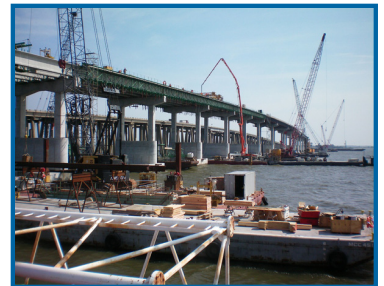
Traylor Bros project, 1.1 mile twin bridges on I-10 over Lake Pontchartrain between New Orleans and Slidell
