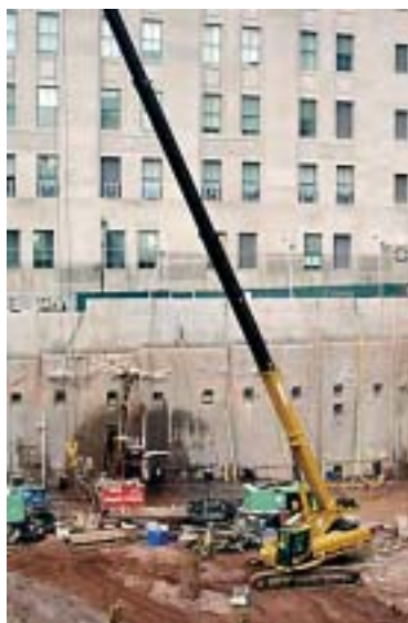
Above: Micropile and Tieback Project, Ground Zero, NYC, NY. Joint Venture: Nicholson + EE Cruz.
