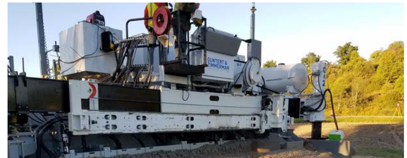
I-390 between Exits 3 & 4 about 12 lane miles of concrete overlay in Central New York
